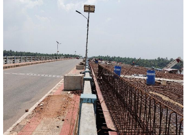
Solar Single arm @ Km 232.830 LHS
