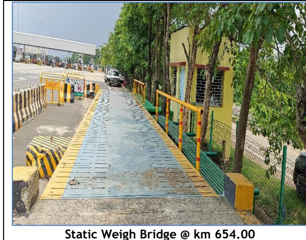
Static Weigh Bridge @ km 654.00
