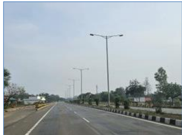
Double Arm Lighting @ Km 182.600 Median
