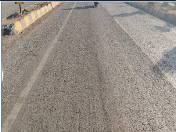
Rutting & Alligator Cracking @ Km 221.500 LHS
