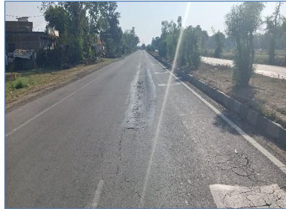
Rutting & Alligator Cracking @ Km 210.000 RHS
