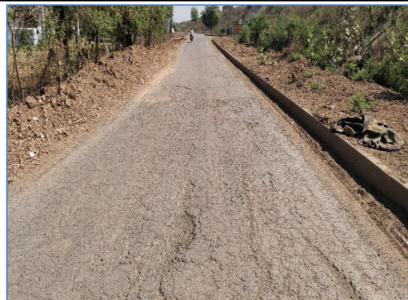
Poor Condition @ Km 222.500 RHS-SR
