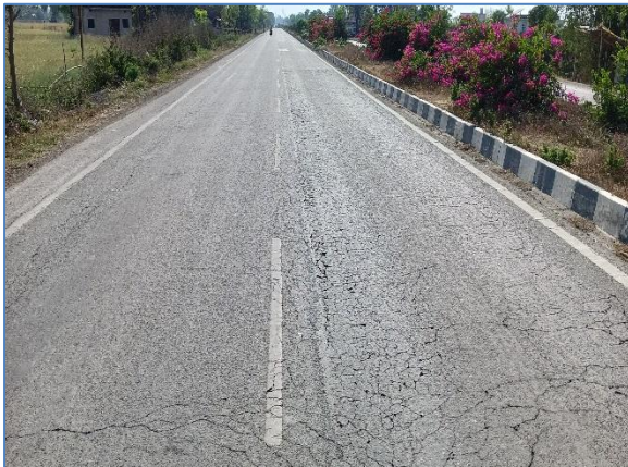
Rutting & Alligator Cracking @ Km 202.000 LHS
