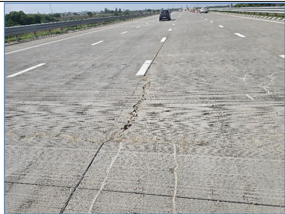
Multiple Cracking @ 298.200 LHS
