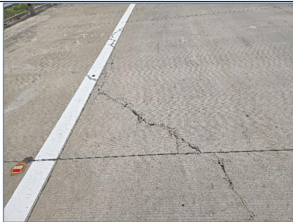
Multiple Cracking @ Km 294.080 LHS
