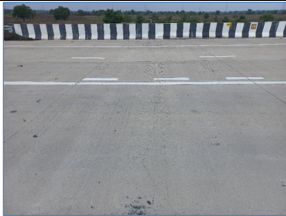
Transverse Cracking @ Km 292.400 LHS
