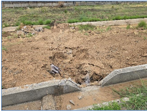
Chute Drain Damage at km 301.700 LHS
