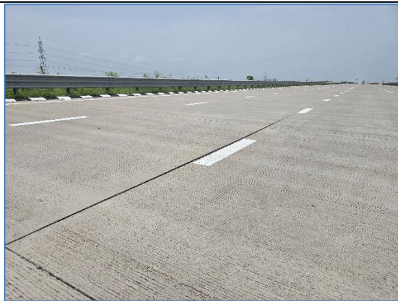
Settlement of Panels @ 308.300 RHS
