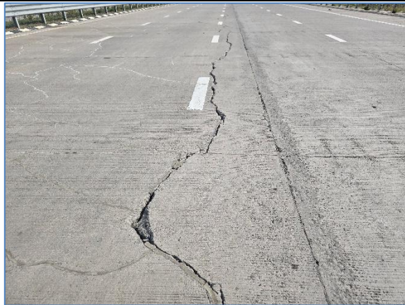
Multiple Cracking @ Km 312.380 LHS
