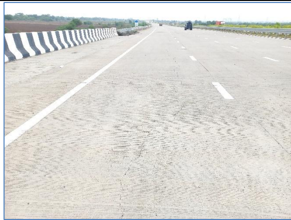
Longitudinal Cracking @ Km 293.450 LHS
