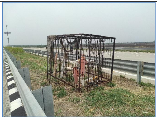
Drip Irrigation Pump @ Km 313.940
