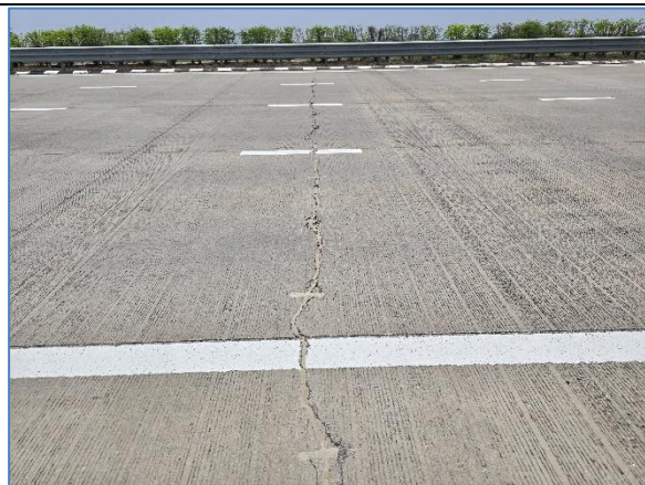
Transverse Cracking @ km311.840 RHS
