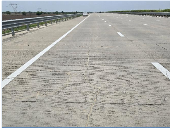
Multiple Cracking @ Km 311.800 RHS
