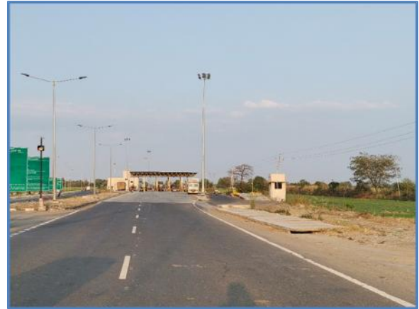
A view of High mast lighting @ km 415.950
