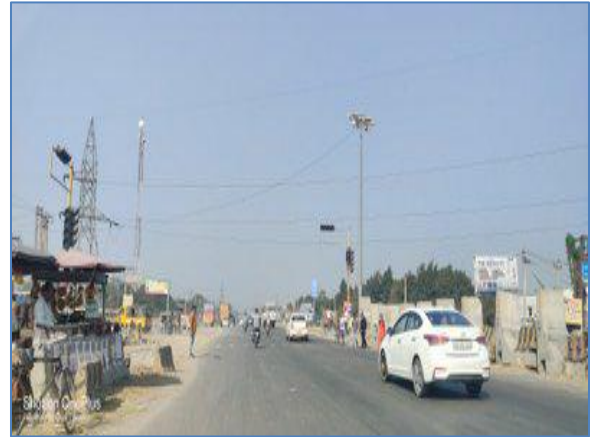
A view of High mast lighting @ km 84.500
