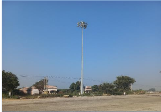
A view of High mast lighting @ km 53.850
