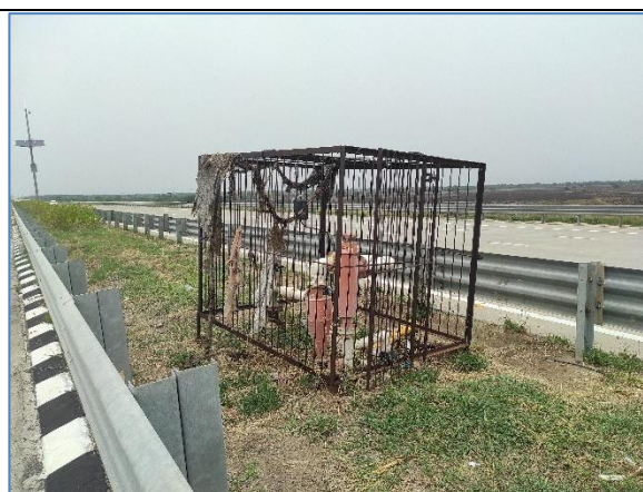
Drip Irrigation Pump @ Km 313.940
