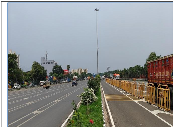
High Mast Lighting at km 654.100 on MCW
