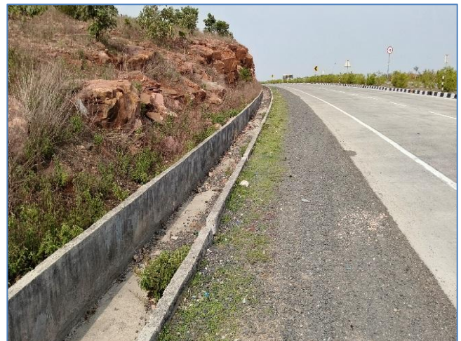
RCC Open Lined Drain at Km 52+300 LHS
