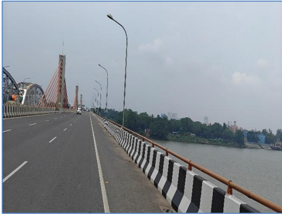
Single Arm lighting at km 657.100 on MCW
