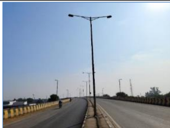
Double Arm lighting @ Km 230.000 Median
