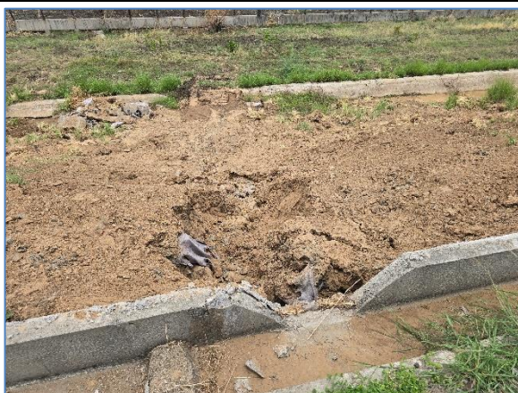
Chute Drain Damage at km 301.700 LHS
